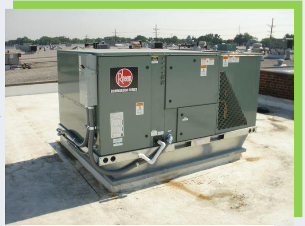
Packaged Heat Pump Unit on Roof
