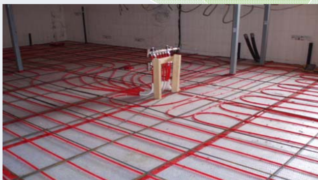
Underfloor Piping System and Manifold
