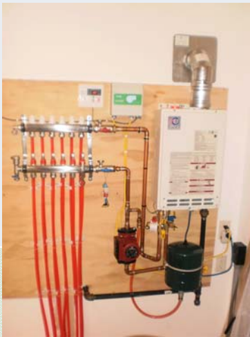
Instantaneous Boiler and Manifold
